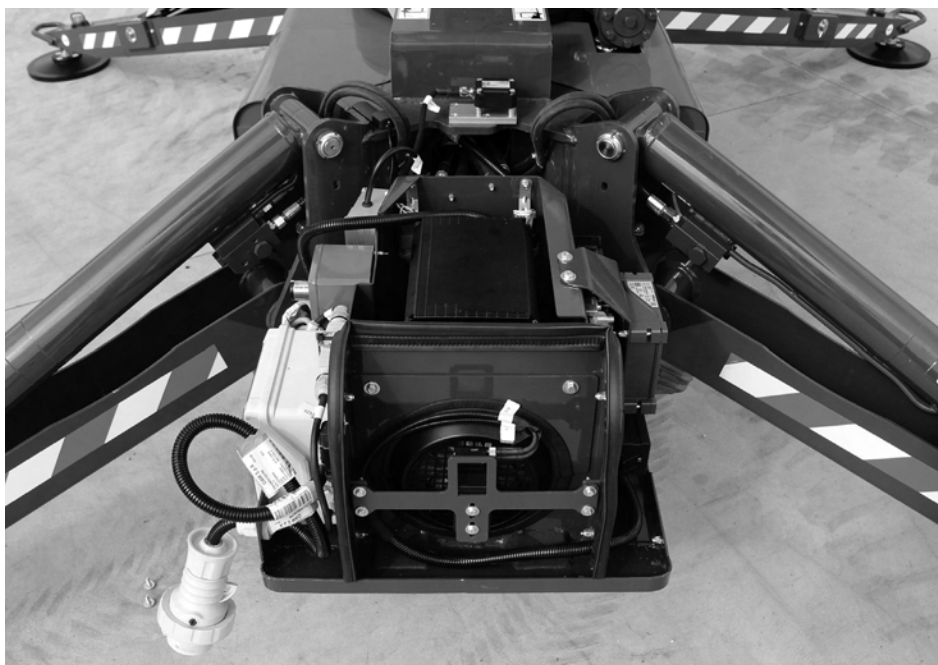
Fig. 153 Electric motor location
