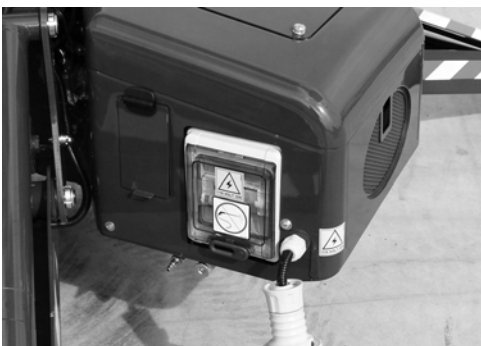
Fig. 80 Main electric switch
